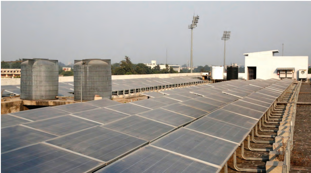
Fig. 11 Solar panel fixed on roof of Thapar Hall building
