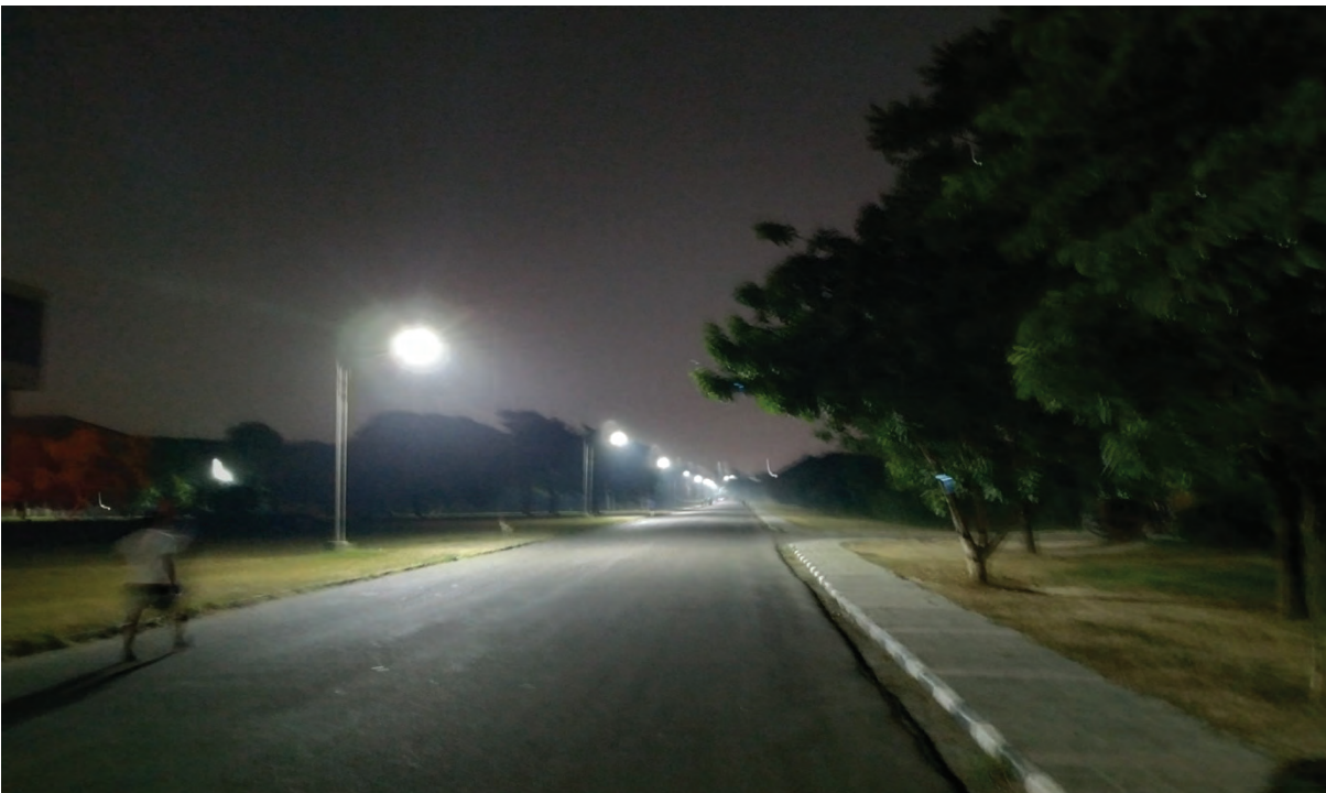
Fig. 12 Led lights in campus
